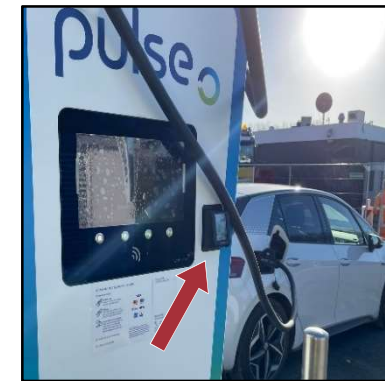
Electric Vehicle Charging Station
